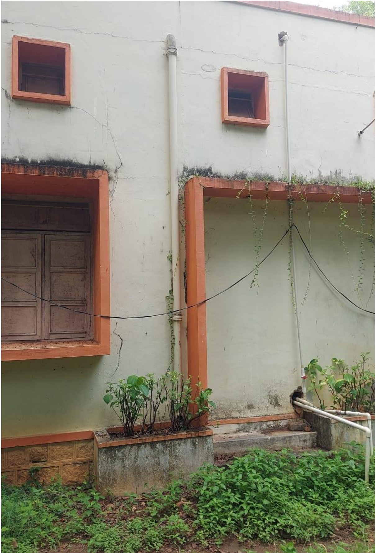
Rain Water Harvesting Roof Top to the Plants
