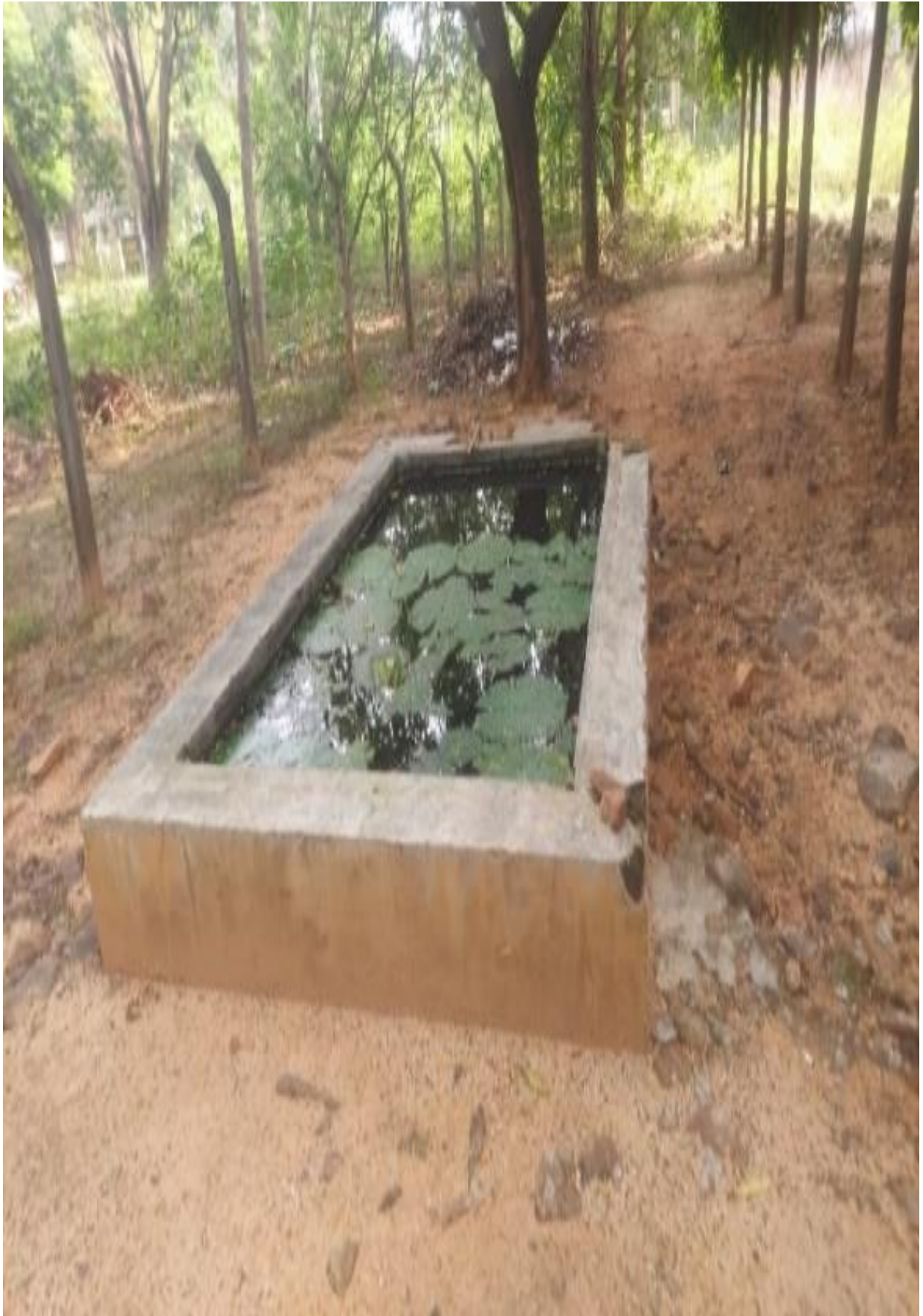
Rain Water Harvesting
