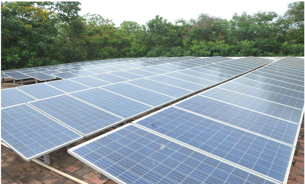
Solar Panel at SVU Hostels
