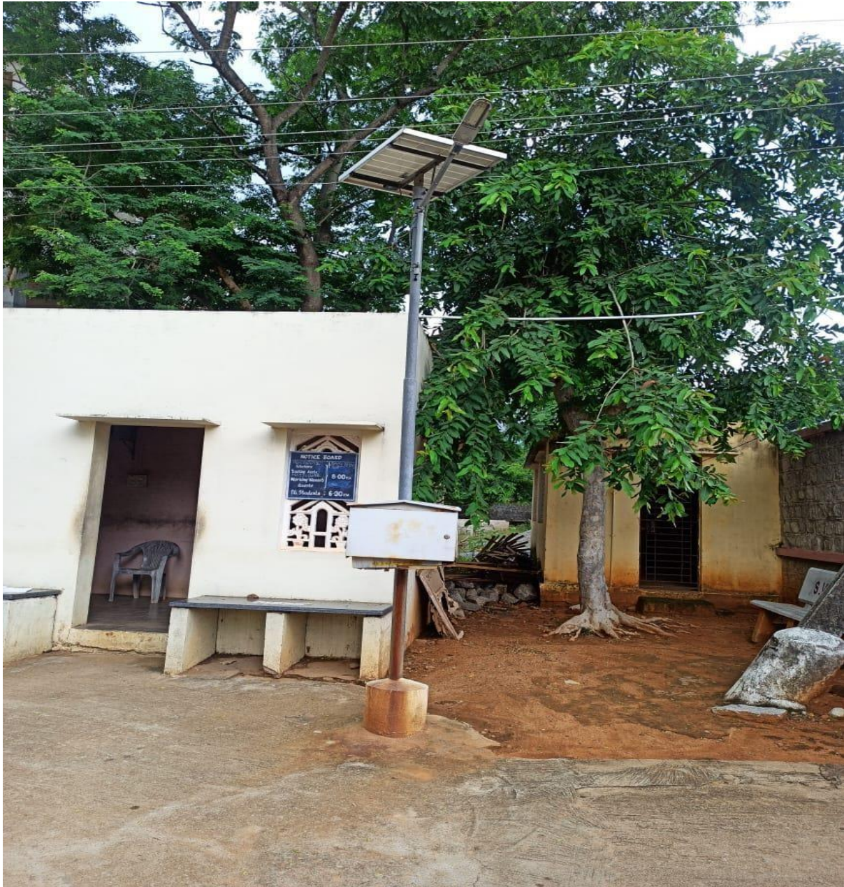
Solar Panels are exported to the Grid of Electricity
