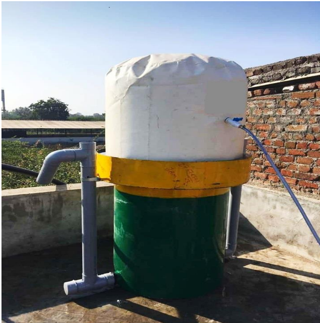
Biogas Plant Facility in the Campus
