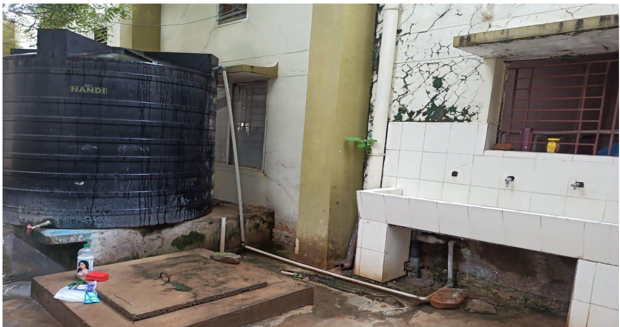
Waste Water Recycling in Women's Hostel
